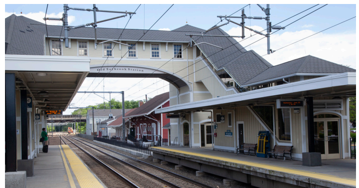
Electric Infrastructure at Old Saybrook Station
